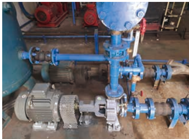
Water Pump Operation
